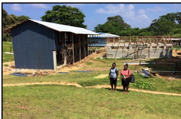
Girls Dormitory and Ablution Block Project at Pawa PSS, Makira taken during a joint project monitoring visit by Procurement and Asset Management Division.
